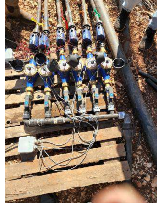
6 irrigation separate controls
